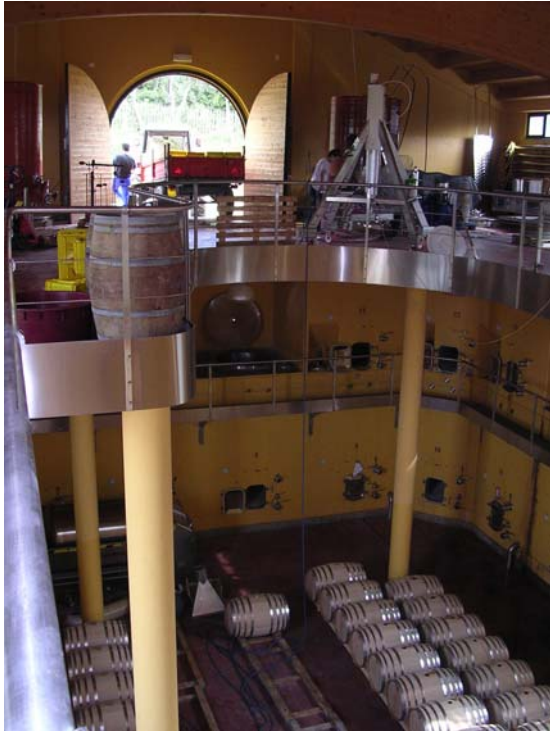
The newly constructed cellar at Caiarossa as the grapes arrive (in tractor at top)
